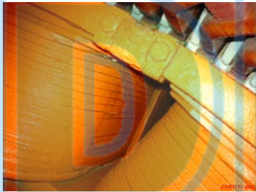
Figure 26: Humidity on the windings
