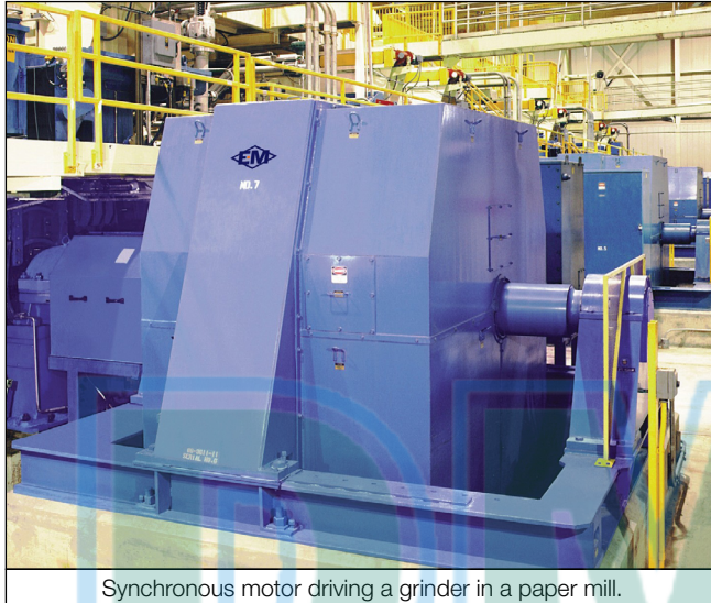
Synchronous motor driving a grinder in a paper mill.
