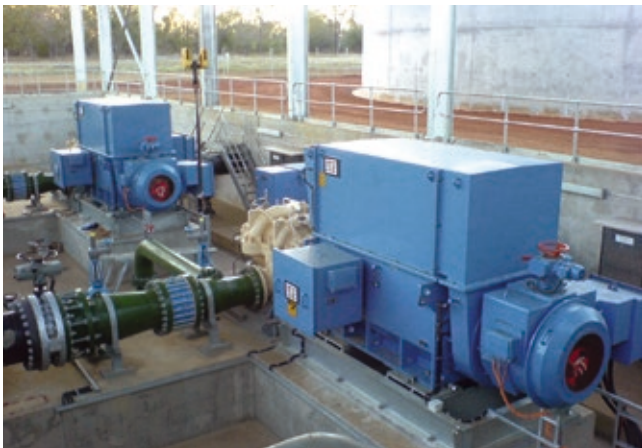
Supply: 2,000 kW, 11,000 V, 4 poles, IC611 Application: Water pump
