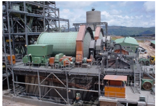
Supply: 6,500 kW, 11,000 V, 6 poles, IC611 Application: Ball mill
