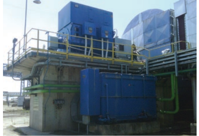
Supply: 9,000 kW, 6,600 V, 8 poles, IC81W Application: Exhaust fan
