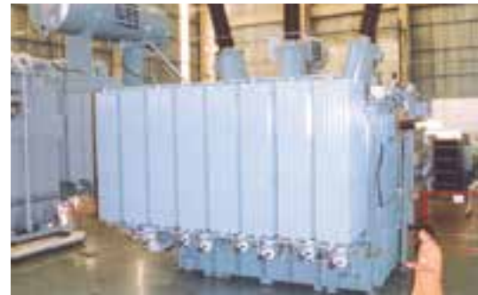
Transformer 60 MVA - 242 kV
