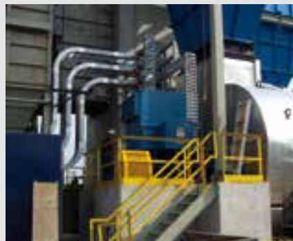
4 x 900 kW, 4,160 V, 8P, frame 8010 (MGP) GERDAU AMERISTEEL - Canada
