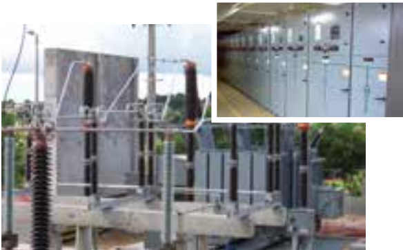
Expansion of the substation CVRD in 242 kV
