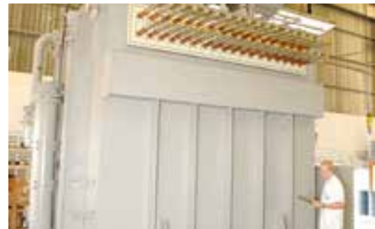
Furnace transformer 75 MVA + 20% - 23 kV, 50 kA
