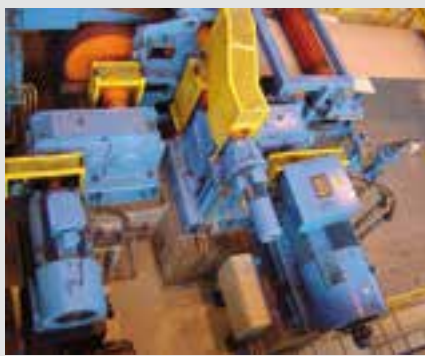
Several Low Voltage motors in VEGA DO SUL (Arcelor Group) - Brazil
