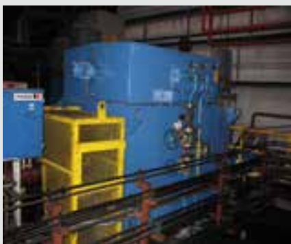
2,000 kW, 8P, VFD Synchronous Motor at SEVERSTALL STEEL PLANT - USA
