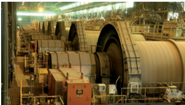
Codelco Teniente Single Pinion Ball Mills - LSS Motors (Retrofit)
