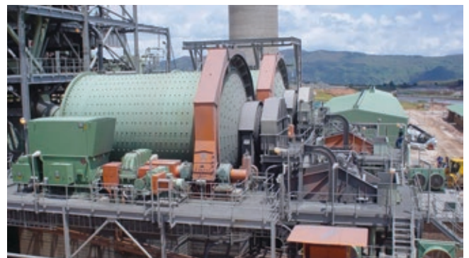
Everest South Platinum Mine Single Pinion Mills: WRIM with Brush lifting device + Liquid Rheostat Starter
